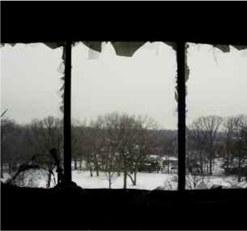
Inside the fire-scarred apartment at Joshua Arms Senior Housing, shortly after the fire.
